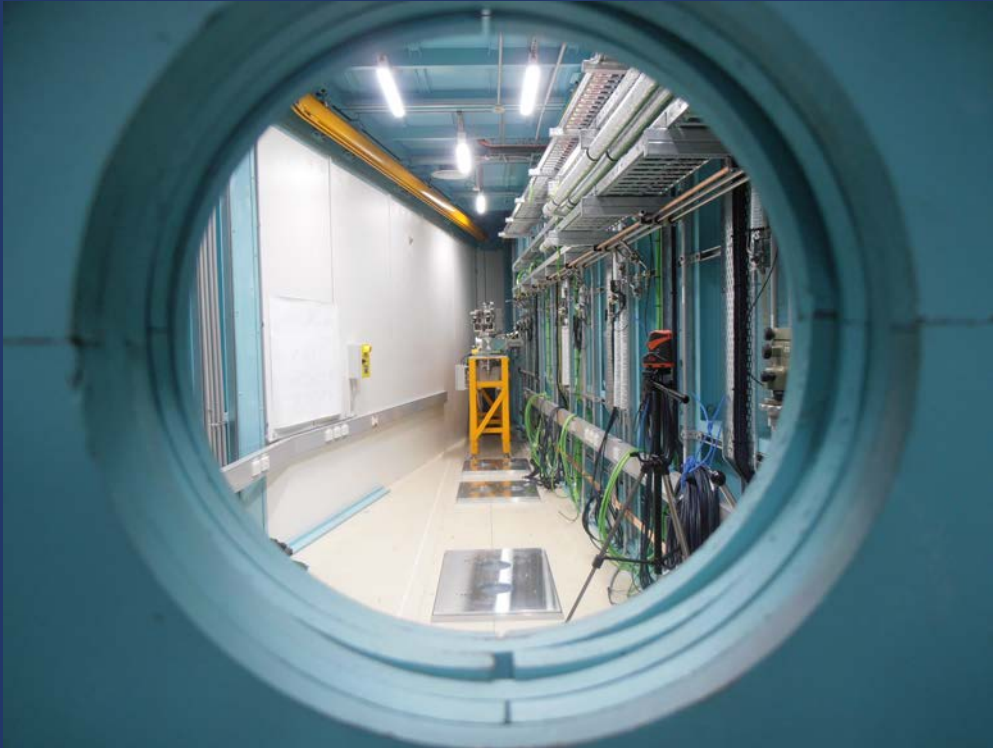
First stand installed at upstream end of MCT first-optical enclosure
