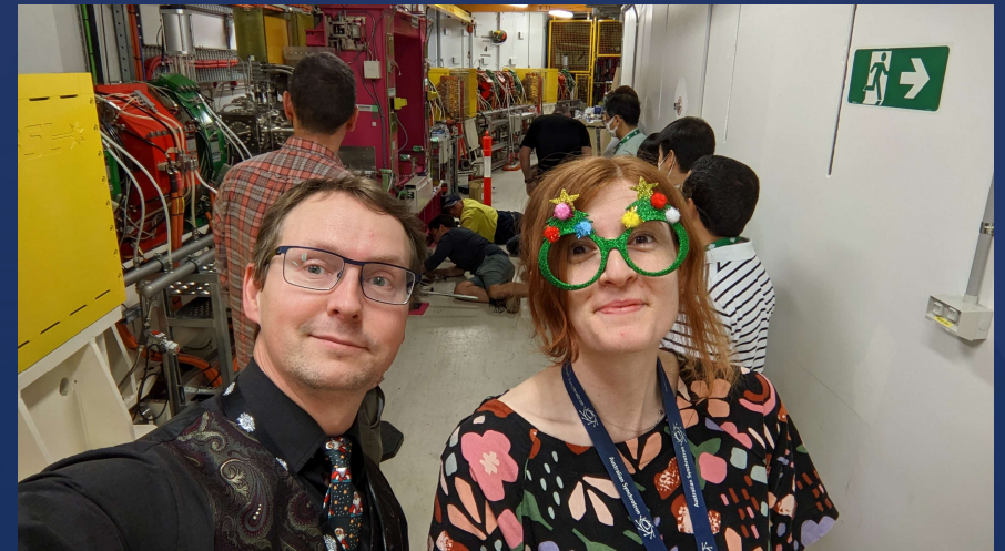
MX scientists' Christmas spirit while expert technicians and engineers install and level the insertion device
