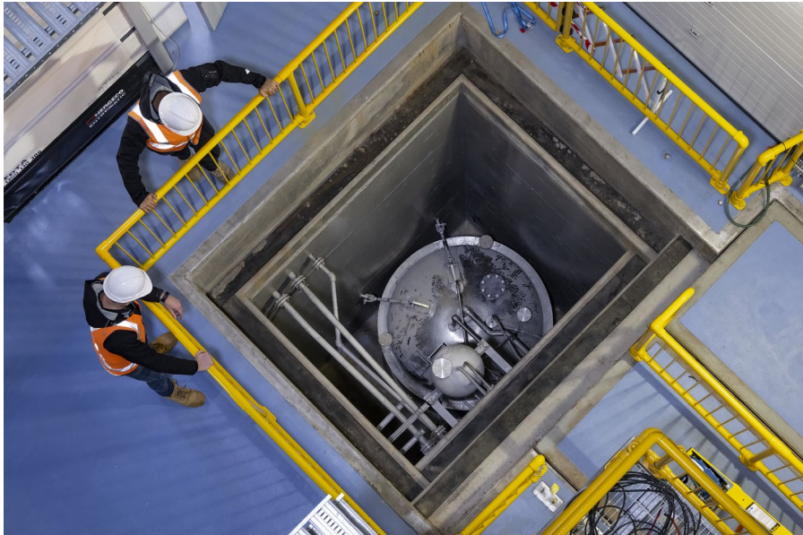
Waste transfer bunker which houses the liquid waste tank in the new ANSTO Synroc® treatment plant, currently in pre-commissioning.
