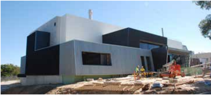
Construction of the new ANSTO Nuclear Medicine facility is now in the final stages.
