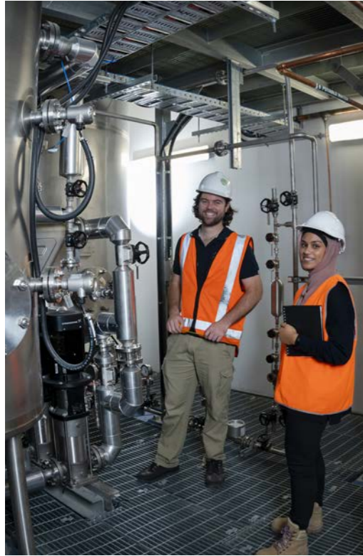
ANSTO employees Brad Davis and Raya Tasnim in ANSTO's first-of-a-kind Synroc Waste Treatment Facility, which is under construction
