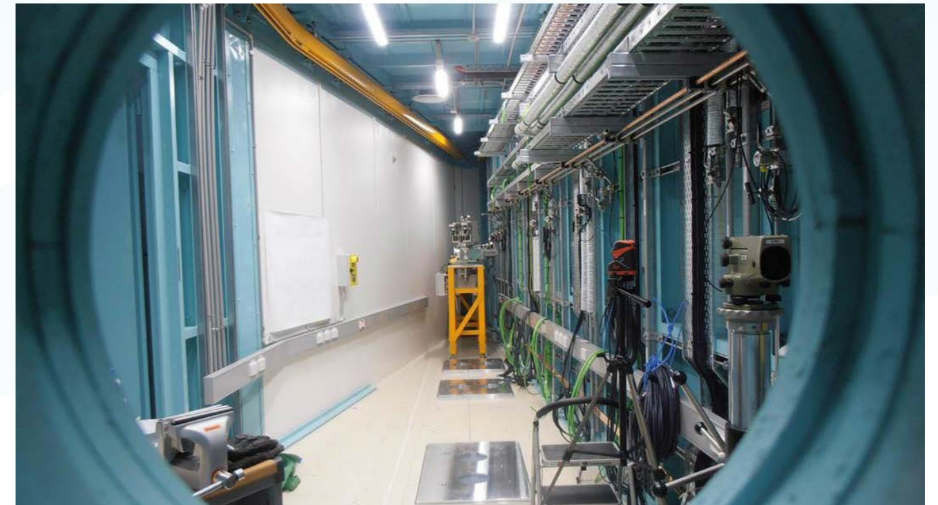
The first-optical enclosure of the Microcomputed Tomography beamline — the view (taken in early July 2021) is looking upstream from the first experimental station
