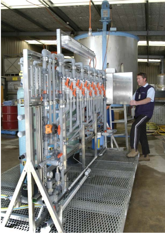
Figure A3 Fixed bed IX rig designed / built by ANSTO installed at ANSTO
