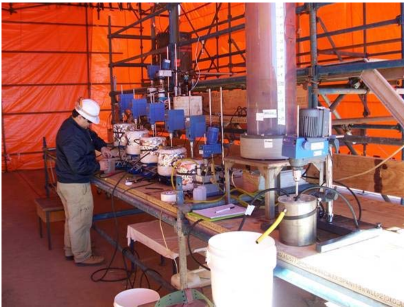
Figure D4 High density sludge (HDS) circuit and high rate thickener designed / built by ANSTO installed on site
