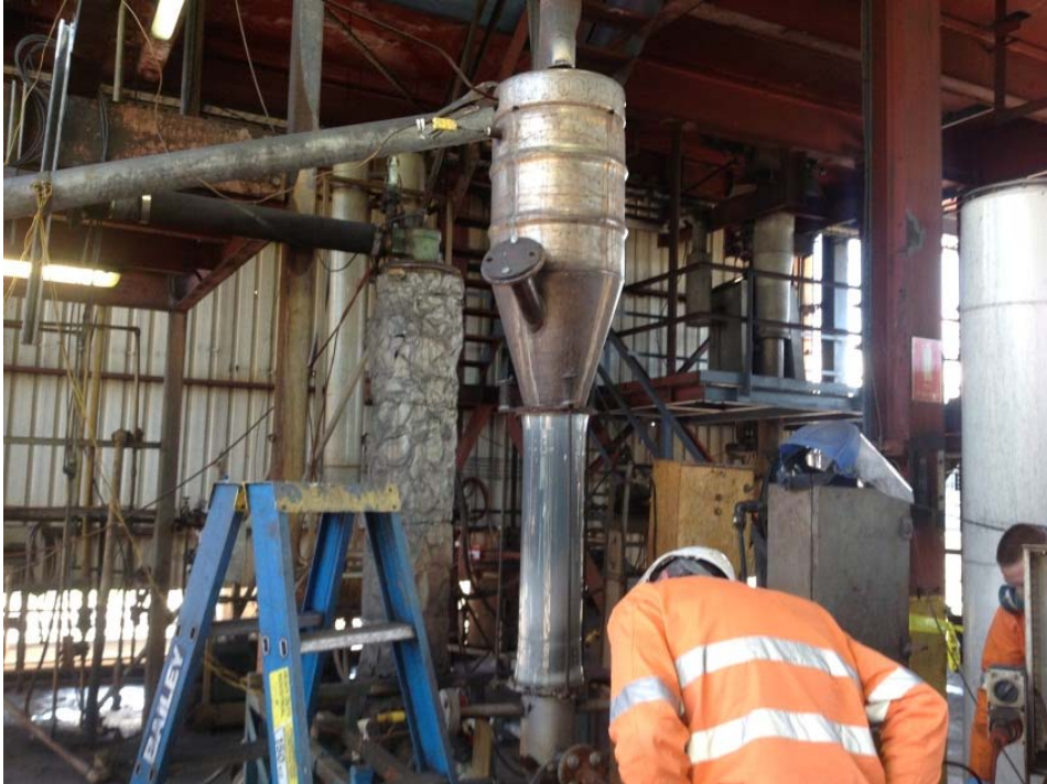
Figure B5 Fluidised bed testing for acid / ore drying / agglomeration on site
