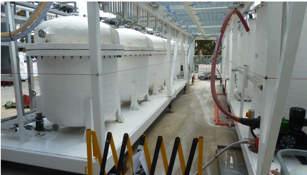
Figure C8 Brine processing demonstration plant at ANSTO –ion-exchange circuit
