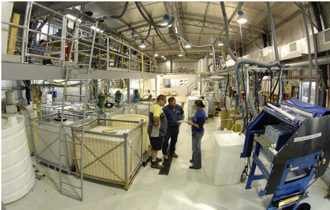
Figure D2 Demonstration plant for Toongi / Dubbo project for recovery of zirconium, niobium, hafnium and rare earths
