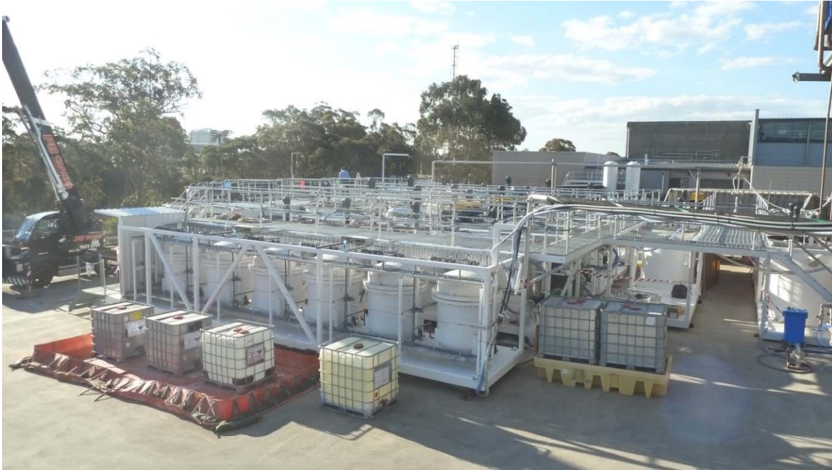
Figure C7 Brine processing demonstration plant at ANSTO – overall
