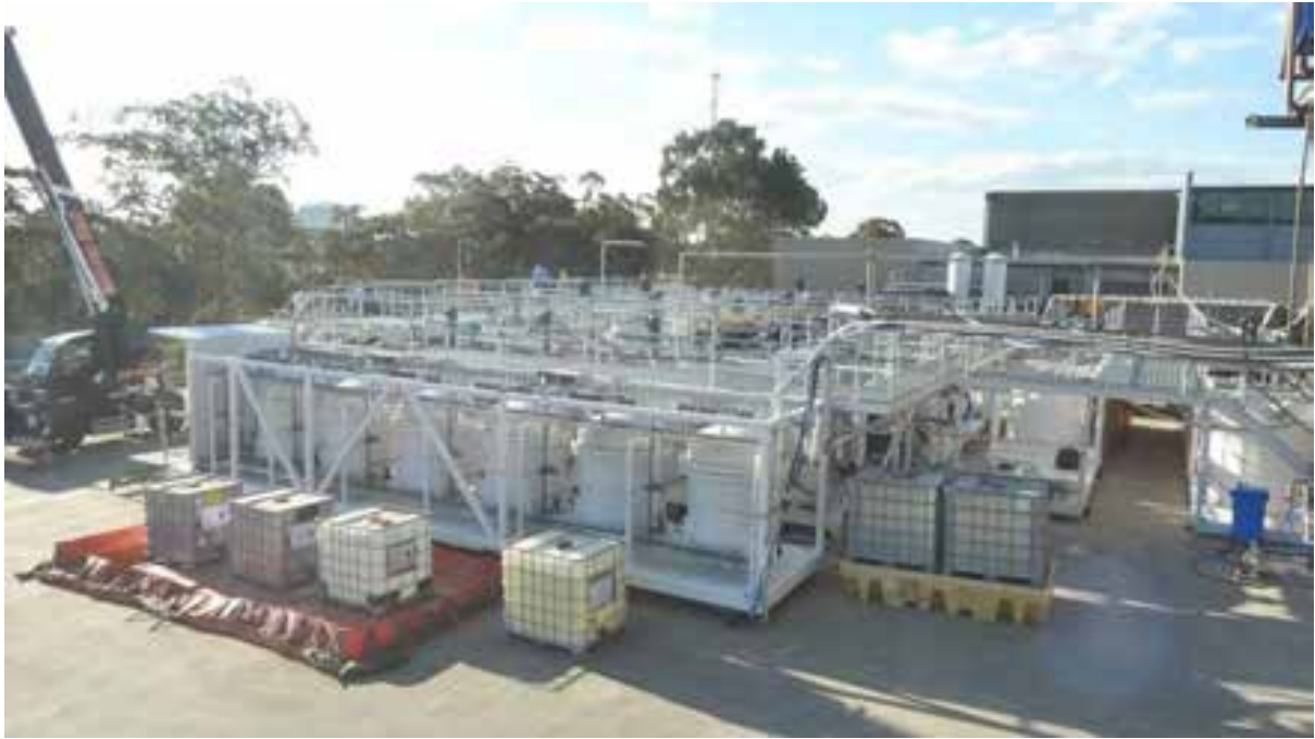
Figure C7 Brine processing demonstration plant at ANSTO – overall
