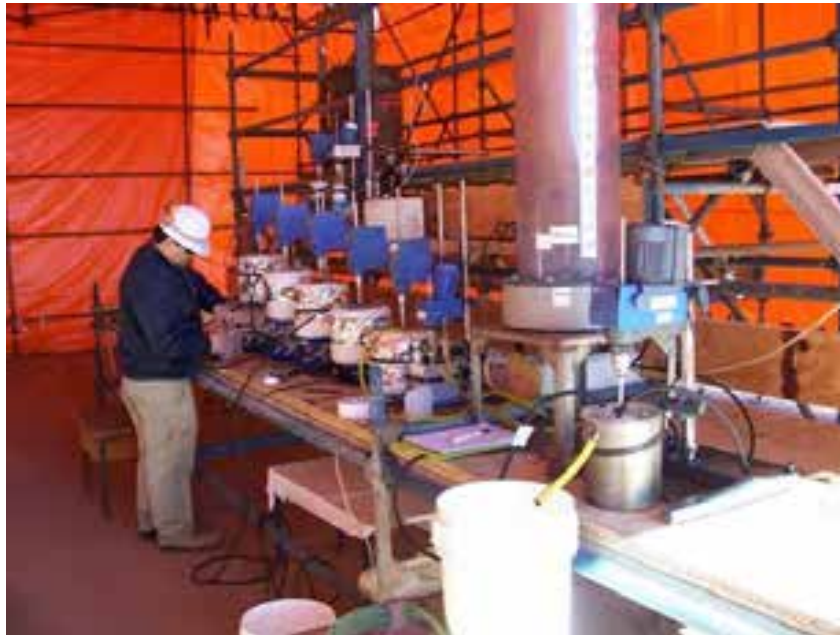
Figure D4 High density sludge (HDS) circuit and high rate thickener designed / built by ANSTO installed on site
