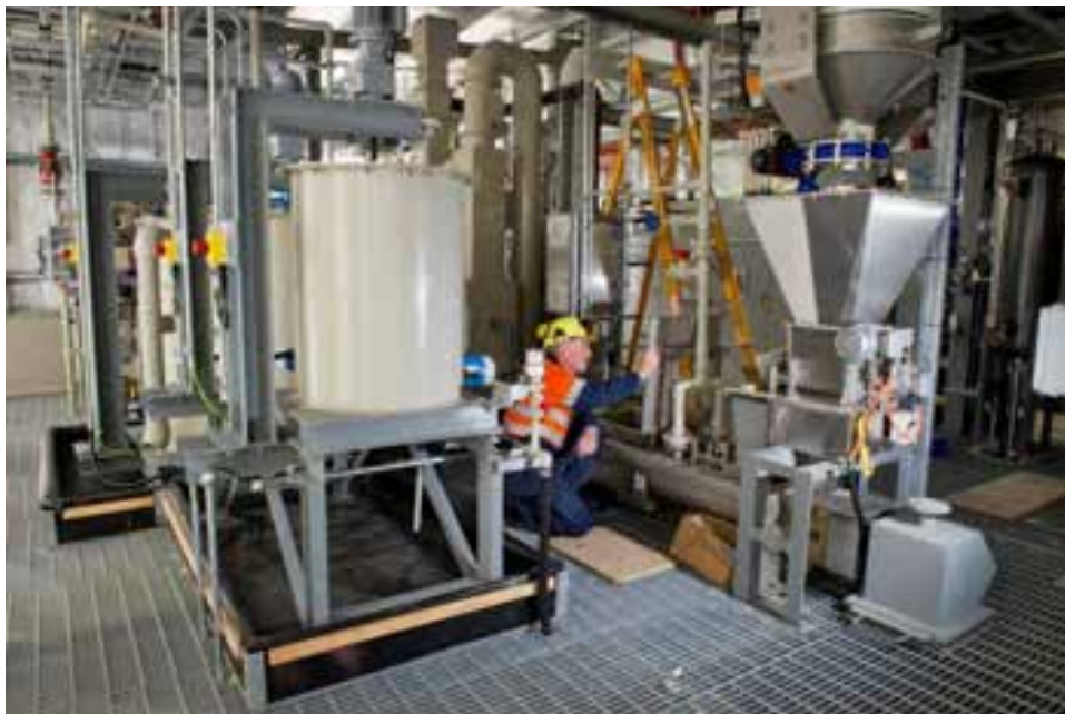
Figure B6 IBS twin-shaft mixer and automatic feed system installed at ANSTO
