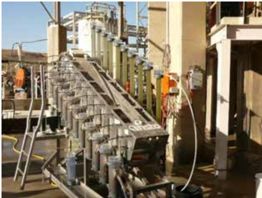
Figure A2 Combined RIP and fixed bed IX rig designed / built by ANSTO installed on site
