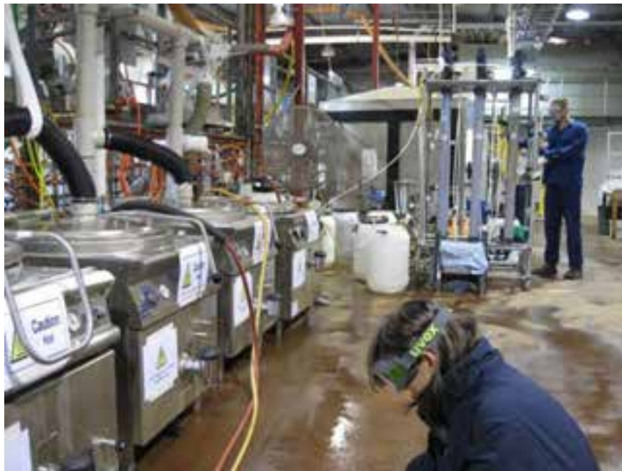
Figure C2 Evaporation and Ca / Mg IX circuits at ANSTO. Up to 20 L/h per unit
