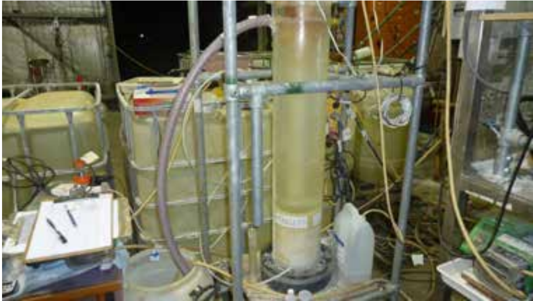
Figure C3 Softening circuit for lithium processing at ANSTO
